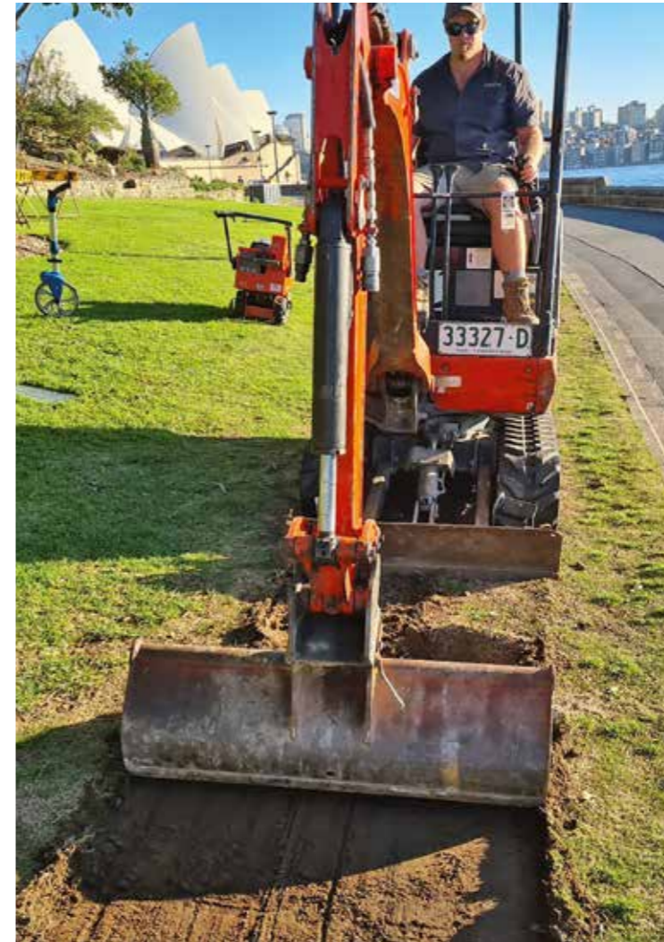
Musturf installing the XtraGrass™ Hybrid Turf System at the Royal Botanic Gardens
